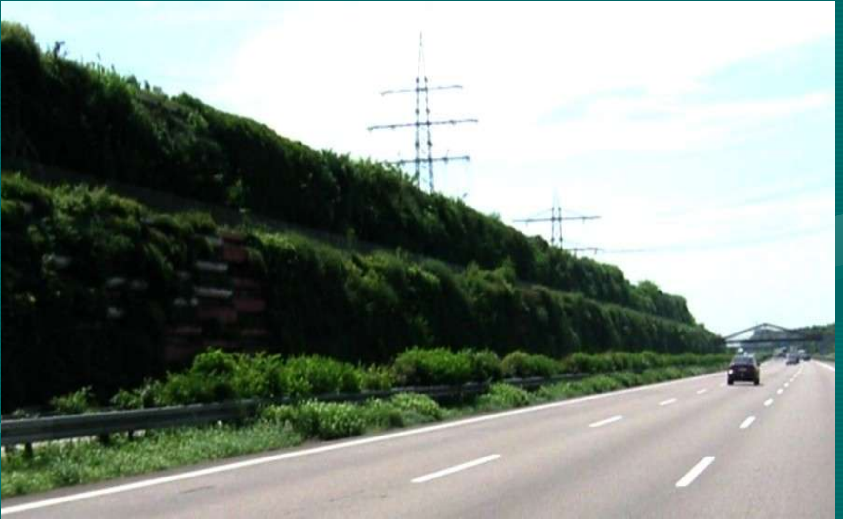
Evergeen GEO near Karlsruhe, Germany
